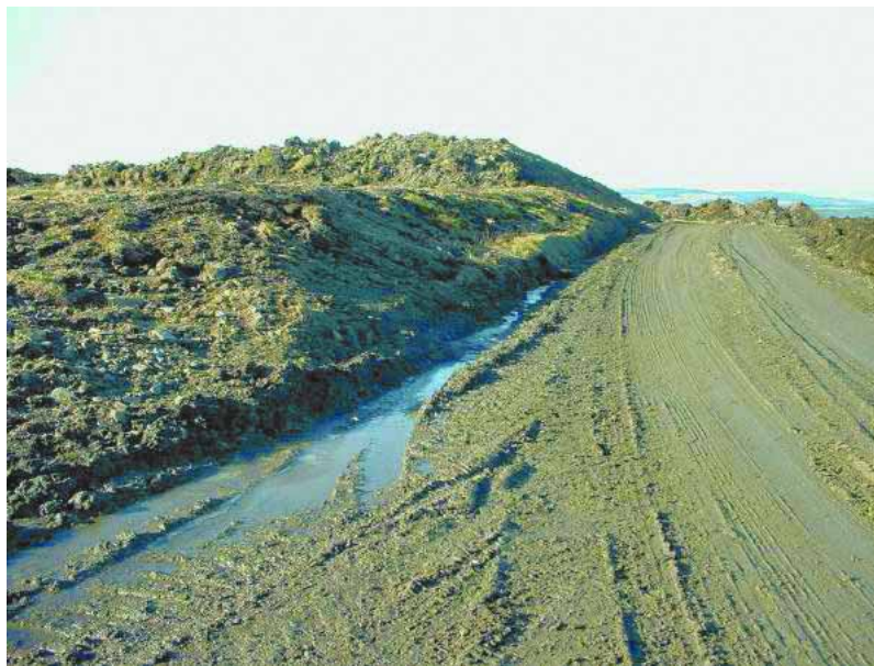
Figure 5: Typical 5 metre wind farm track with collateral damage extending to the sides at the Ffynnon Oer wind farm, Vale of Neath
