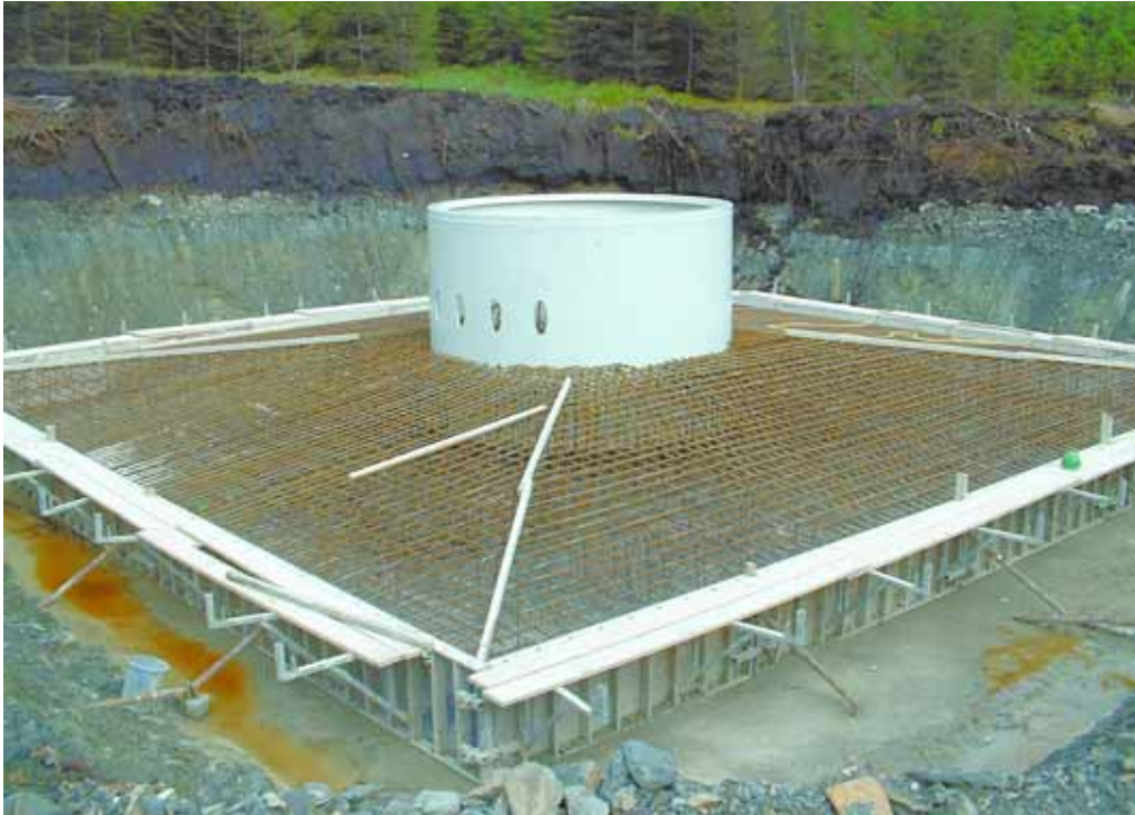
Figure 8: Wind turbine base at Cefn Croes, Wales, showing steel reinforcing bars and collar in place prior to pouring concrete. Note the 2m deep peat cut through at the rear.
